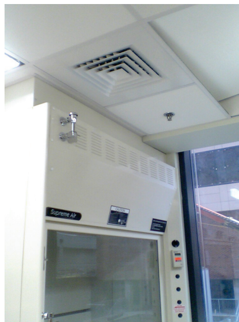
Figure 14. Diffusers blowing air at fume hoods can cause turbulence, hindering containment.
