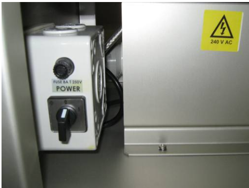
Figure 12 – Power switch location
